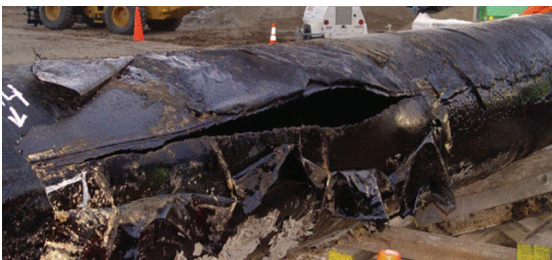
Ruptured 6B pipeline - Kalamazoo, Michigan, 2010
